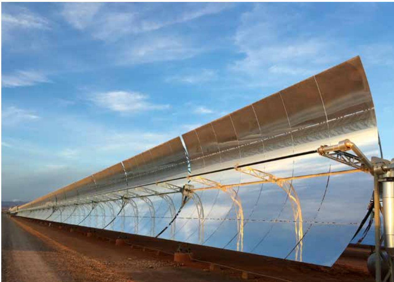
The Nour solar plant near Ouarzazate in the Moroccan desert uses more than half a million parabolic mirrors to generate power. Morocco is increasingly becoming a renewable energy leader.
